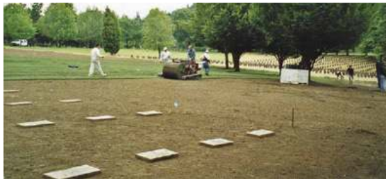
Renovation of Willamette National Cemetery where Pro Landscape replaced more than 1 million square feet of sod.
